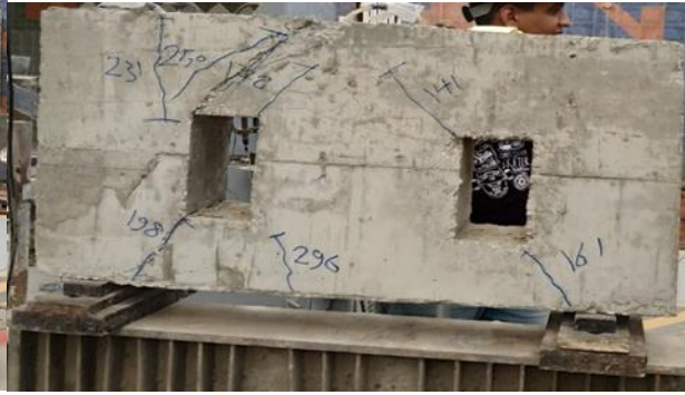
B3-RO-V: Diagonal-shear splitting failure
